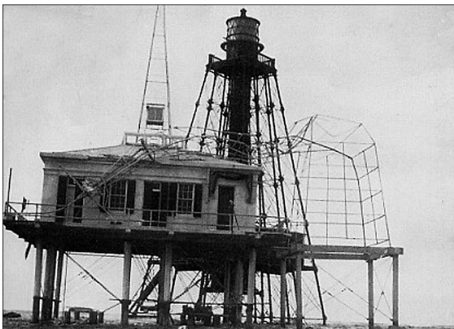
Sand Key in 1919 showing the hurricane damage. The antenna is collapsed on the weather station. Photo courtesy of the author.
