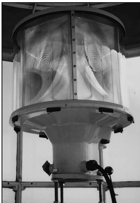
Left – The new Vega optic installed in the lantern room of the Sand Key tower. This new type optic is manufactured in New Zealand and used around the world. Photo courtesy of the author.
