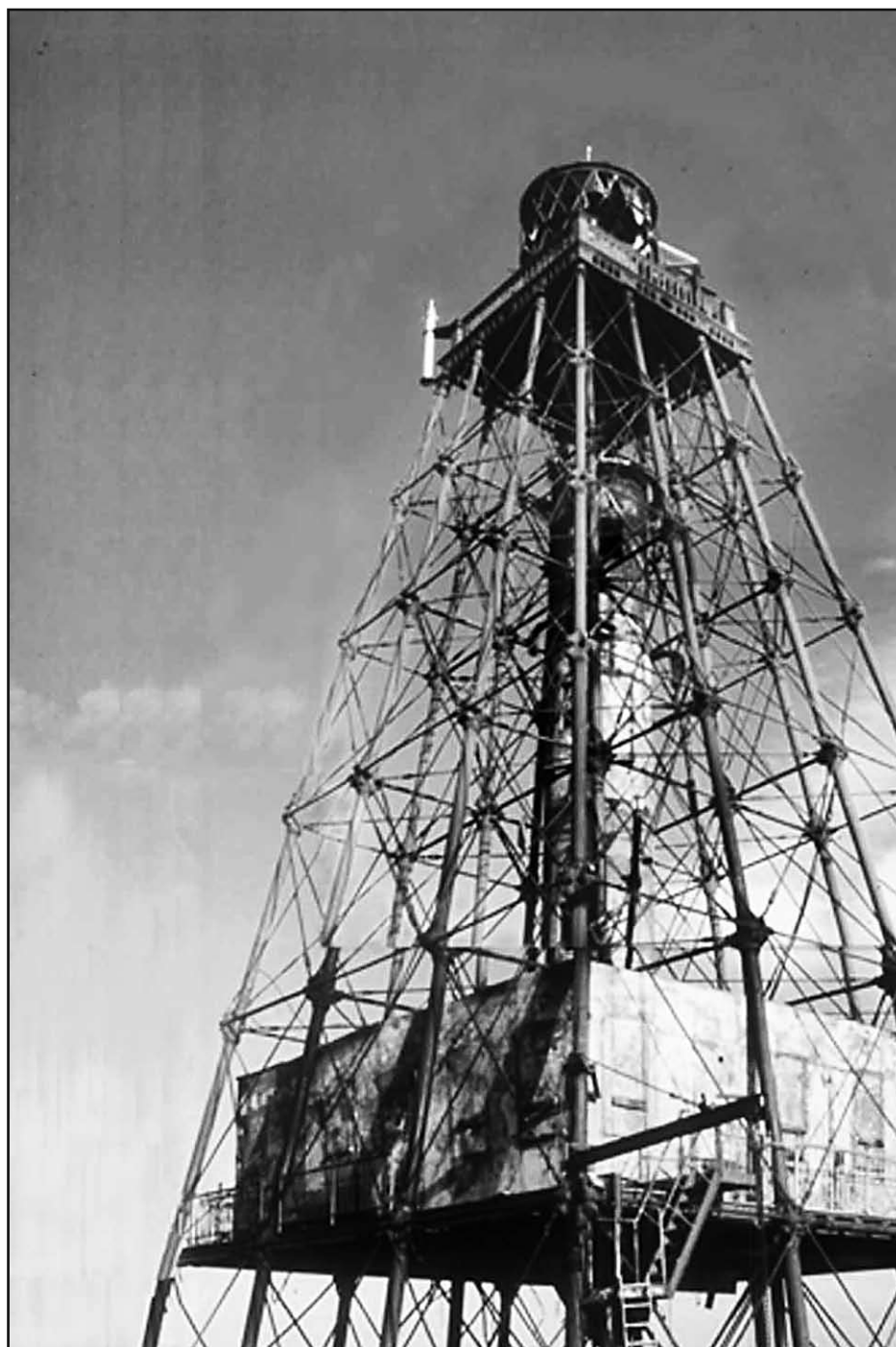
View of the damage to the Sand Key tower. Photo courtesy of the author.
